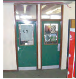
Door and glass above a door (Risk Code 1 & 5).
